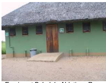
Erosion at Babalala Ablutions Ramp
